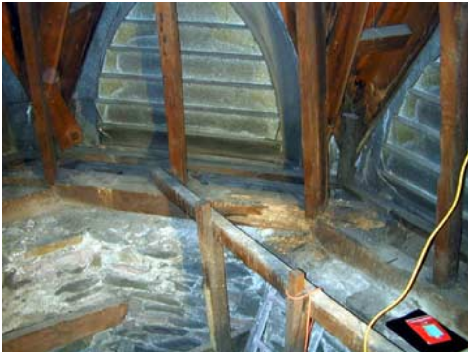
Figure 022: East Tower - Photo showing additional area of dry rot at intersection of two sill plates and vertical spire support
