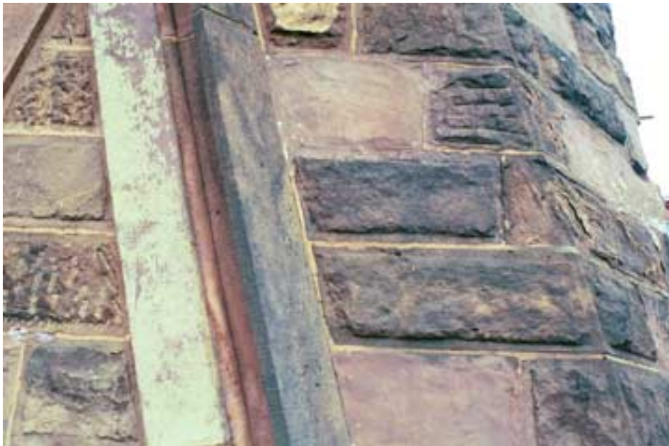
Figure 004: Photo showing area of similar patching as well as delamination of the sandstone façade on surrounding stones (Notice the hard edge of the mortar where inappropriate mortar was used in earlier repointing campaign)
