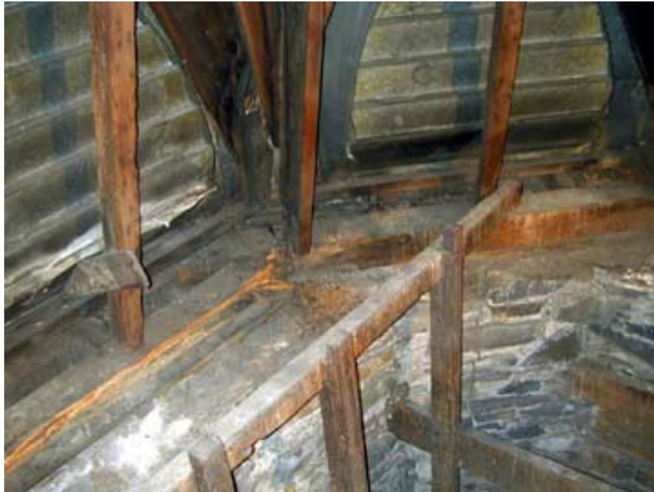
Figure 019: East Tower – Photo showing area of rot running the length of the sill plate
