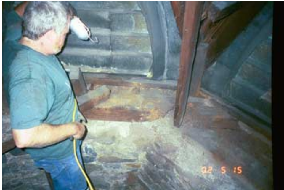
Figure 024: West Tower - Photo showing total failure of sill plate at intersection of vertical support and lapping sill plate (for adjoining section)
