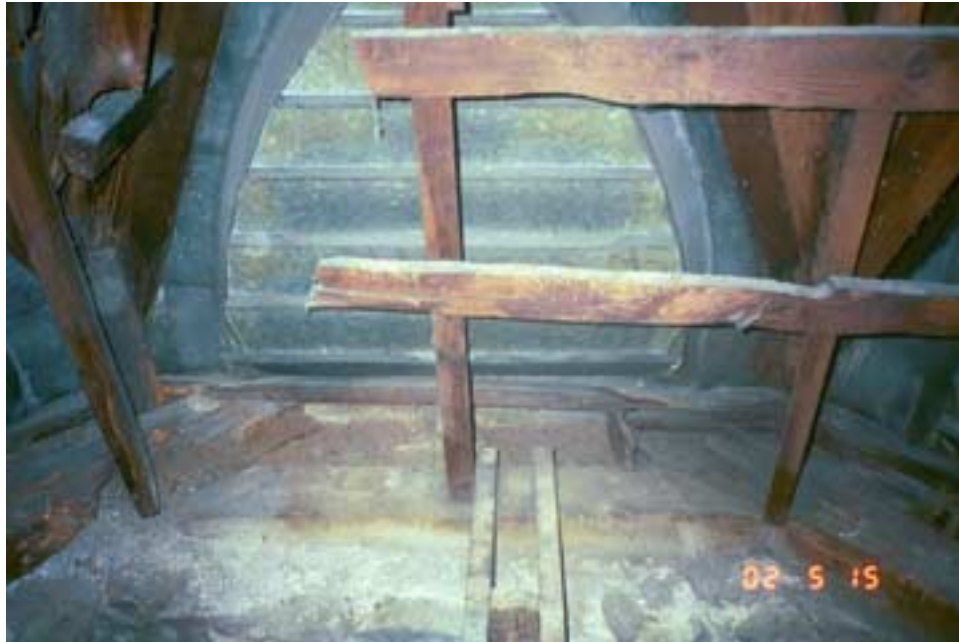
Figure 027: West Tower - Photo showing failed sill plate, lap joint (left), galvanized decorative exterior without any ventilation capacity, deteriorated one-by material
