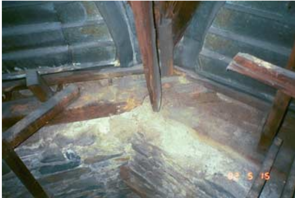
Figure 025: West Tower - Photo showing failed lap joint of sill plate (typical)
