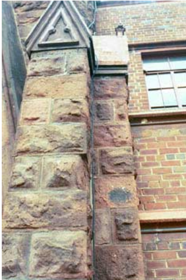
Figure 007: Photo showing area of relatively sound stone next to the administrative offices; however, selective stones continue to show deeply eroded surfaces secondary to weakened facades
