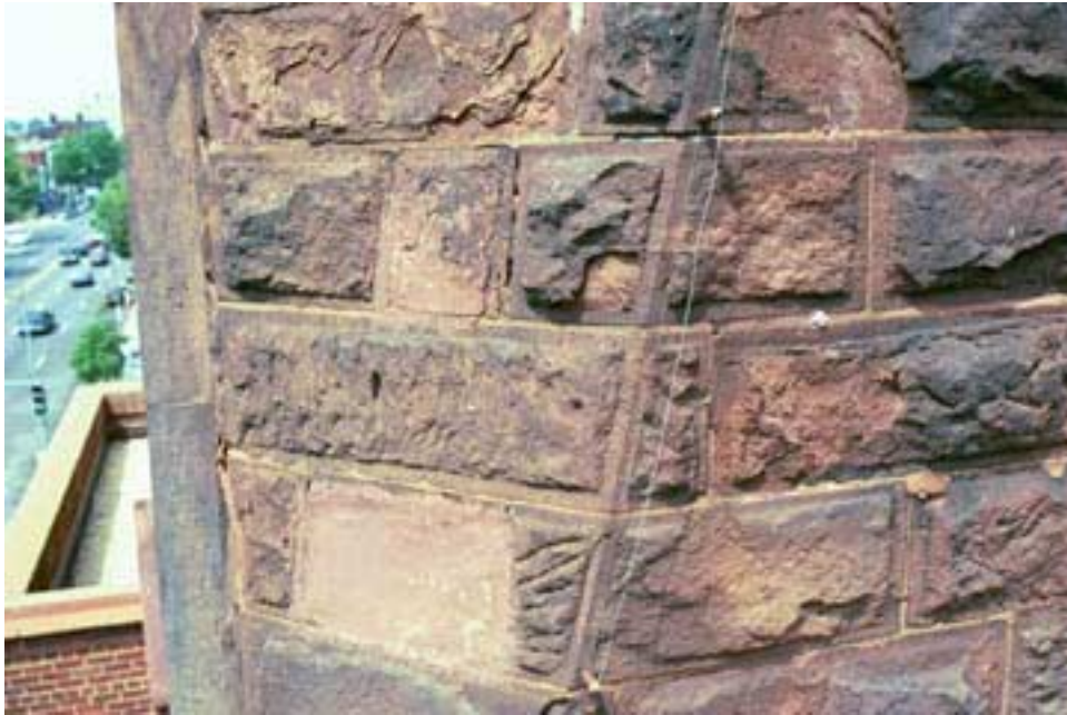
Figure 003: Photo showing area of cementitious patching and penetrations created during earlier campaign to control pigeon population.
