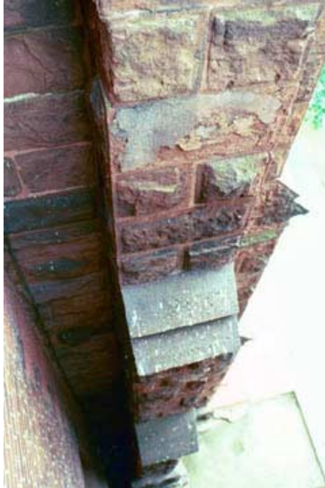
Figure 006: Photo showing areas of delaminating sandstone façade, and presence of large quantity of pigeon guano
