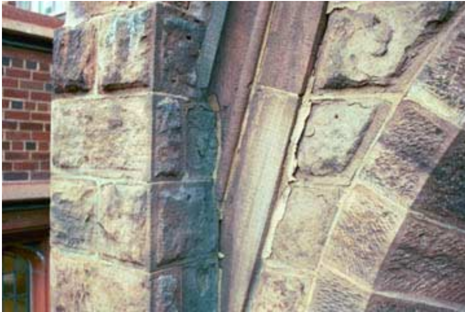
Figure 001: Photo showing area of mortar loss and subsequent failed repair
