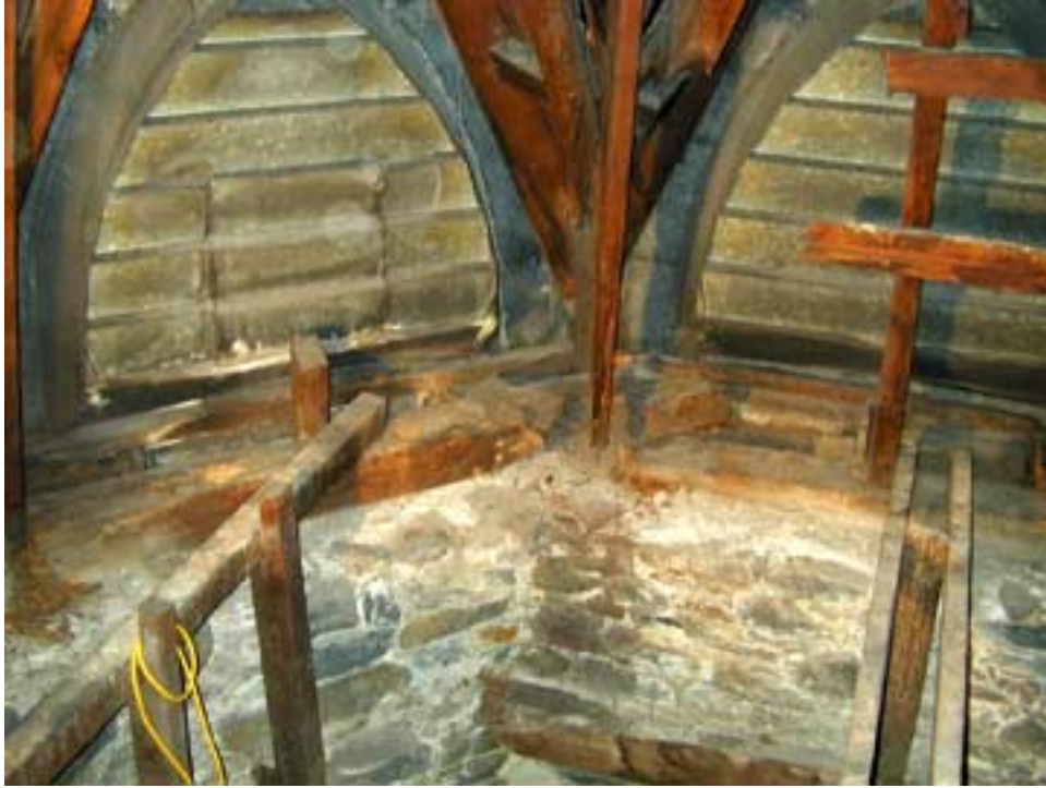
Figure 021: East Tower- Photo showing dry rotted sill plate and location of onetime opening into tower loft.
