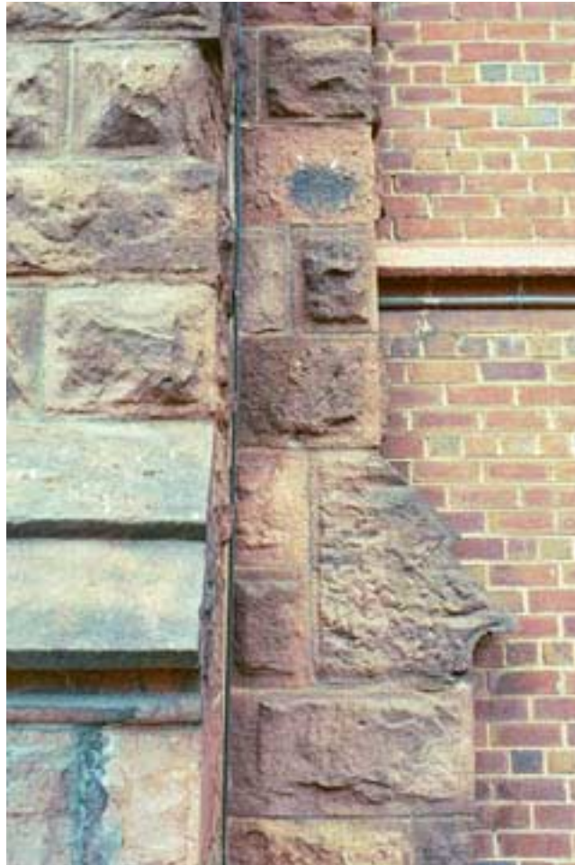
Figure 008: Photo showing areas of stone that are performing well (Condition of walls improves closer to the ground with most of the significant damage at the very peaks of the two towers.)
