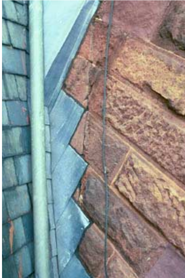
Figure 014: Photo showing close up view of flashing detail (note exposed reglet and heavily applied tar/caulking along edge of new flashing.)
