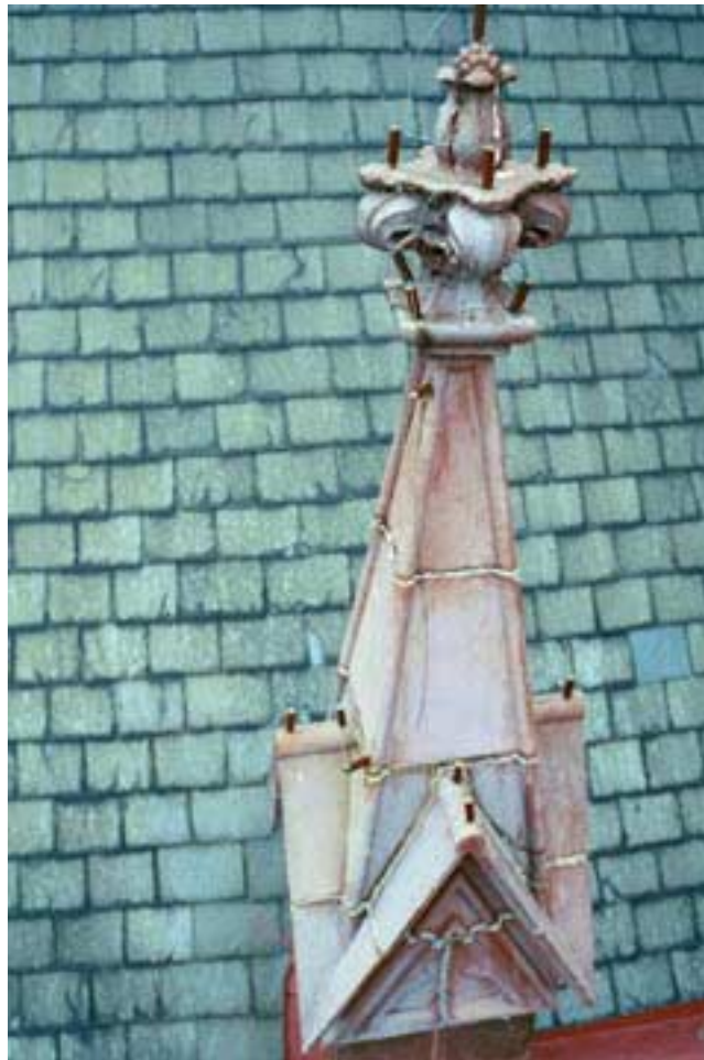
Figure 011: Photo showing terracotta minaret with multiple penetrations and superficially applied caulk over mortar base (need to determine stability of each minaret and need to repair as necessary)
