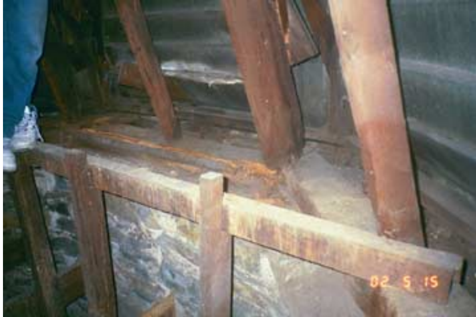
Figure 023: West Tower- Photo showing sill plate with rot and decay sufficient to compromise the entire length of the plate from vertical support to vertical support. Intermediate support is resting on hollowed out sill plate as well thus provided no additional vertical support for spire along exposed façade.
