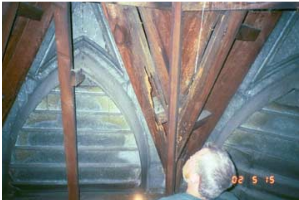
Figure 030: West Tower - Photo showing area of compression damage caused by loss of vertical support at corner of spire (damage has been compounded by insect infestation and dry and wet rot)
