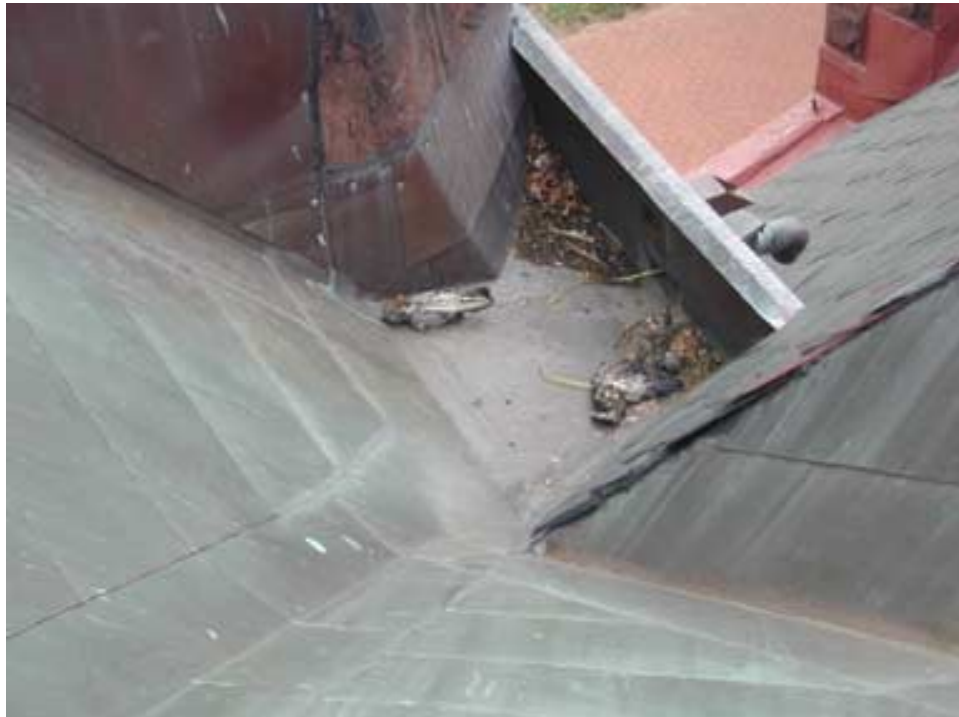
Figure 018: Photo showing general condition of roof drainage system at base of tower spires
