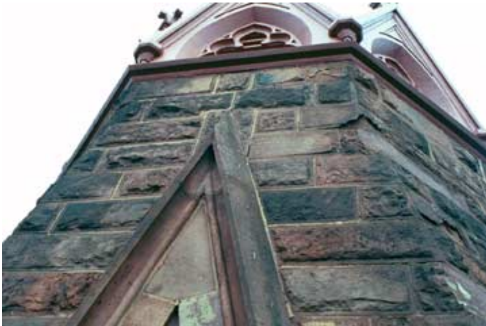
Figure 002: Photo showing area of large sections of failed mortar joints typical of both towers above the level of the first floor
