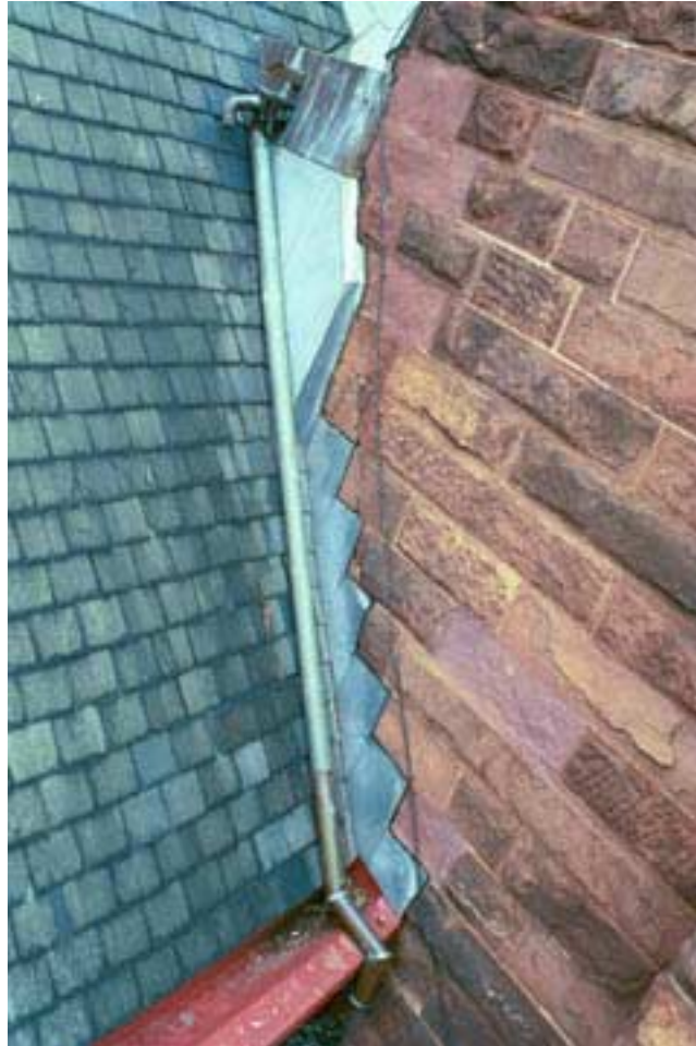
Figure 013: Photo showing flashing at intersection of roof and east tower: Flashing detail is highly irregular with efficacy difficult to predict.
