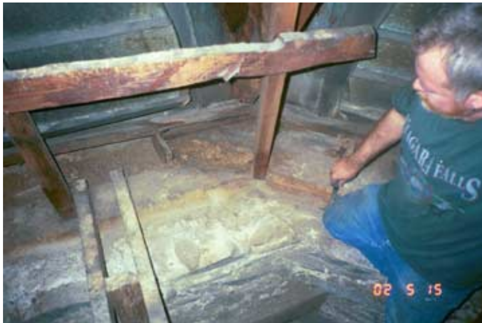
Figure 026: West Tower - Photo showing failed lap joint at sill plate (typical)
