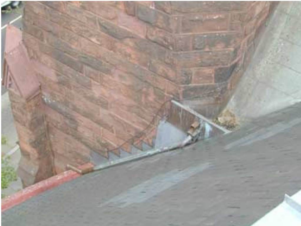
Figure 016: Photo showing large amount of nesting material at drainage collector: This atypical drainage and overflow system does not appear to meet any typical set of specifications for such work and should be rethought (southwest face of west tower)
